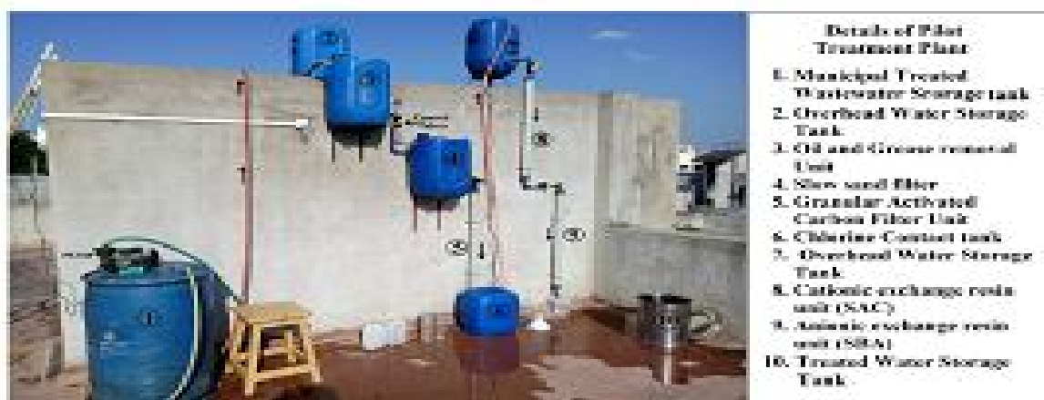
Fig 1: Photograph of actual pilot treatment plant
